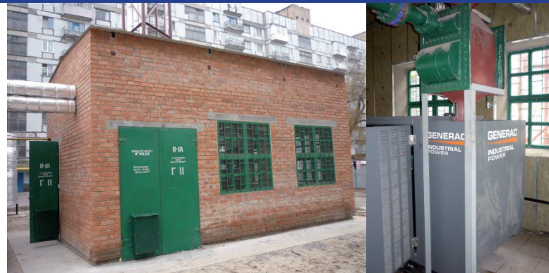
Reconstruction of the CHS-room into mini-CHP
